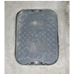
Floor plate cover for backwater valve.
